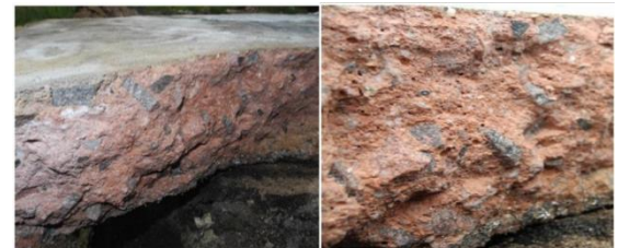
Figure-2. Chemical Decomposing of Concrete.
