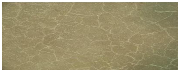
Figure-1. Surface Cracks
