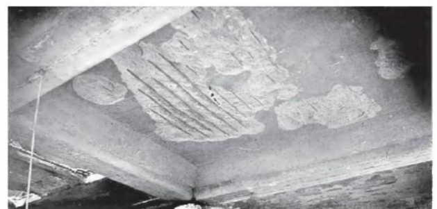
Figure-3. Spalling of the concrete cover during a moderate fire.
